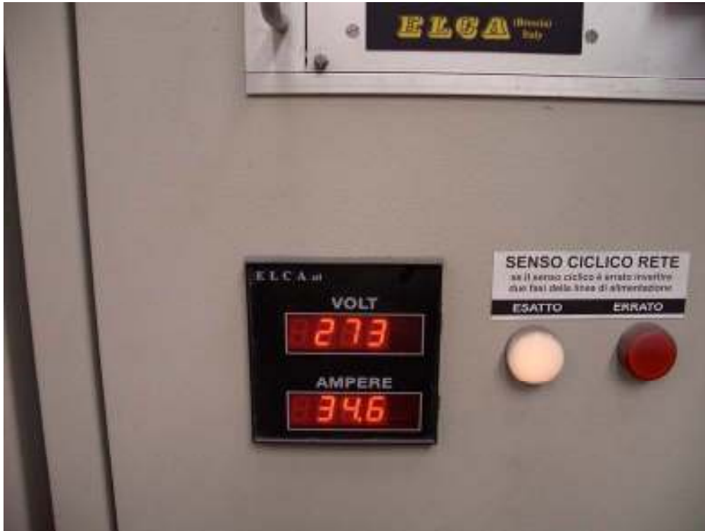
Figure 27 – Particular of the control board of the current supply almost at the end of the process. The full control board is shown in figure 24.
